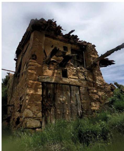
Fig.7 Study of degradation phenomena and structural pathologies (Source: Authors).
