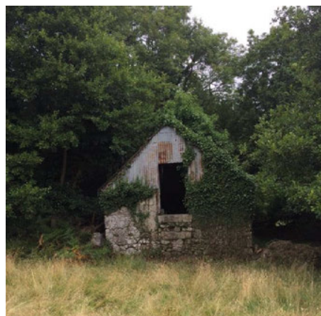
Fig. 3. Beckhams Linhay south gable before repair (Source: Jonathan Rhind Architects, 2019).
