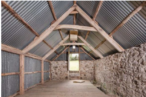
Fig. 4. Beckhams Linhay. Tallet interior looking south following repairs (Source: Copyright Historic England Archive, Davies, 2021).
