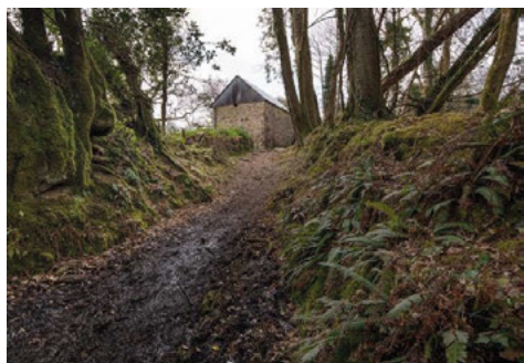
Fig. 2. Beckhams Linhay. North elevation following repairs (Source: Copyright Historic England Archive, Davies, 2021).
