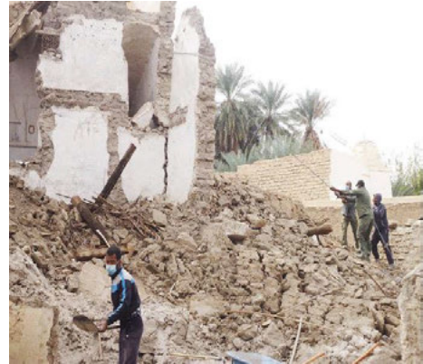
Fig. 9. Disaster due to excessive rainfall.
