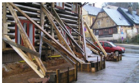
Fig. 1. Façade of the pub “Dřevěnka Inn” No. 92 (house formerly) supported by interim oblique back shores with balk and stone footing that is secured by iron anchor rods in the drilled opening, Úpice Village, Trutnov District, Hradec Králové Region © Martin Cernansky, 2008, NHI
