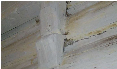
Fig. 5. House No. 53 built of logs used for walls and ceiling. Apart from this profiled bracket, there are also simple shape brackets under the supporting beam. Rtyně v Podkrkonoší Village, Trutnov District, Hradec Králové Region © Martin Cernansky, 2008, NHI
