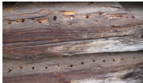
Fig. 6. Watermill No. 2 (82) and improving material properties using resin injection, Zubrnice Rural Reservation, Ústí nad Labem District, Ústí nad Labem Region © Martin Cernansky, 2015, NHI
