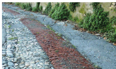
Fig. 4. Cambered profile of the central brick strip and lateral cobble-stone channel (Source: Fratini).
