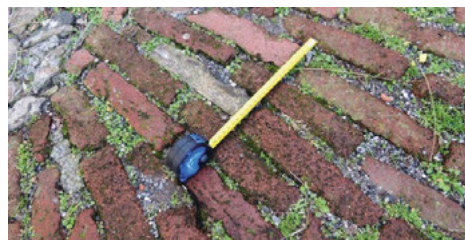
Fig.9. Old bricks with a rough appearance, with a slight tendency to disintegrate (Source: Fratini).
