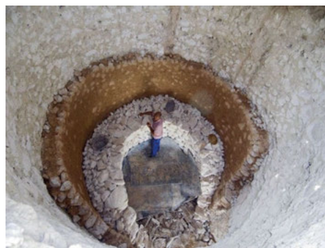
Fig. 3. Construction of the lime kiln, Morón de la Frontera, Sevilla (Juan Carlos Cazalla, 2008)
