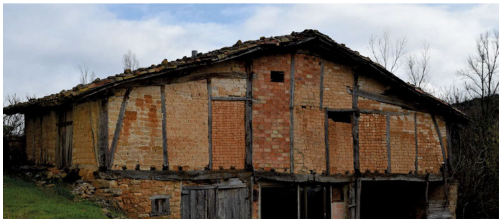
Fig. 2. Building in Villanueva de Tobera (Burgos), showing material lesions (damp stains, erosion, loss of volumetry, rot, replacement of infill, elimination of structural elements) and structural lesions (excessive buckling of timber, lack of bonding and fissuring of the infill) (Source: Hueto-Escobar, 2022).
