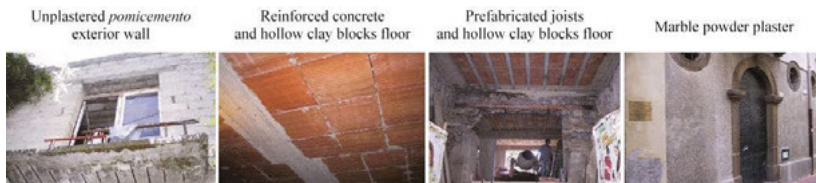
Fig. 3. Examples of inappropriate interventions on vernacular Aeolian architectures (Source: the Authors)
