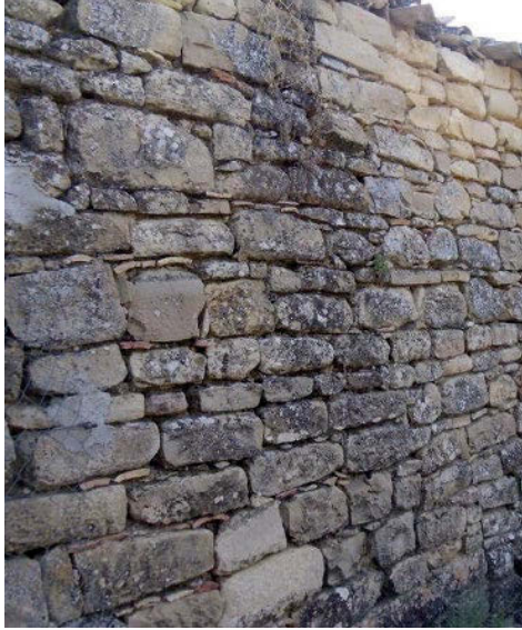
Fig. 4. Detail of a wall in Porcuna without mortar ( a hueso construction). (Source: Belmondo, Millán, 2022).
