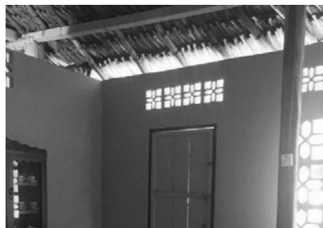
Fig. 3. Roof expansion over the wall, space for exit of hot air. (Source: Authors, 2021)
