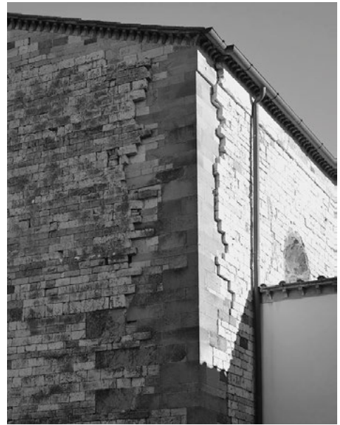
Fig. 3. damage to the wall caused by the earthquake in 1542. Church of Sant'Agata, Mugello (Source: Bordoni, 2021).
