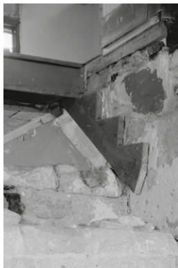
Figura 55: Restos de escalera interior. Fuente: Historic American Buildings Survey, C. (1933) Don Raimundo Arrivas House, 44 South George Street, Saint Augustine, St. Johns County, FL. St. Johns County Florida Saint Augustine, 1933. Documentation Compiled After. [Photograph] Retrieved from the Library of Congress, https://www.loc.gov/item/fl0198/s
