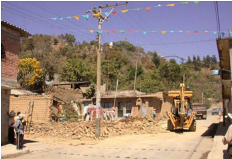
Fig. 9. Adobe houses ordered to be demolished against people's will (Source: Aguilar Prieto, 2001).
