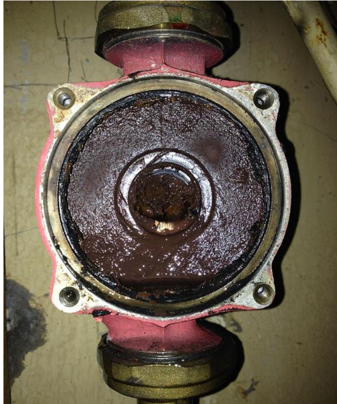
Figure 2.10: Circulation pump blocked by contaminants (Janlepkowski, 2014)
