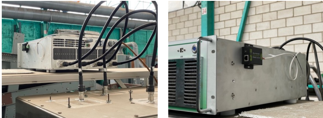
Fig 8.32. Modbus ethernet converter external installation.
