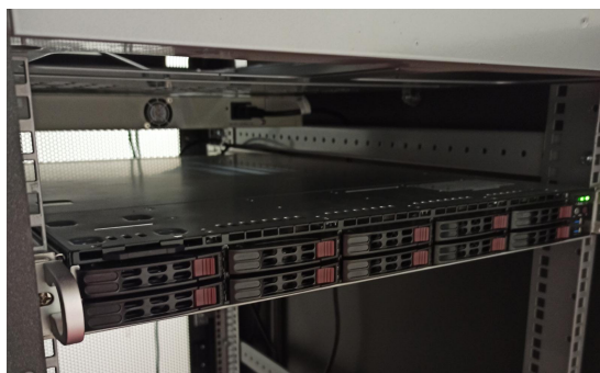
Figure 4.6: The SuperServer 1029P-WTRT, which hosts several 5G Cores and Network Functions and is the foundation of the Open 5GC Laboratory
