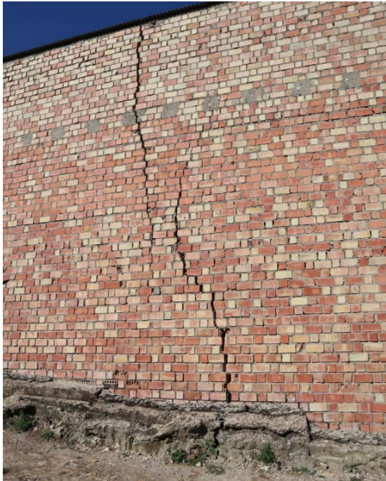
Figure 8. Cracks in a build from the southeast shoulder sector. The wall shown is oriented N160°E (north to the left), the observed displacement being strictly parallel to this orientation.
