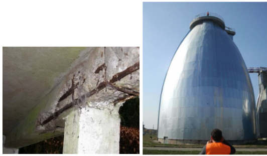
Figure 2. Concrete structures, where deteriorations are critical.
