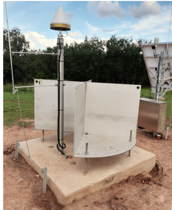
Figure 4. RAG's MSST for Saarland's SaarBoBeKa. Left: reinforced concrete foundation 2m x 2m x 2m, lightning rod, JAVAD RingAnt-G3T GNSS chokering antenna, D-CR \varnothing 2,0 m and levelling points in foundation and D-CR. Right: solar power supply, weather sensors, mobile radio antenna, equipment box. Image courtesy ALLSAT & RAG.
