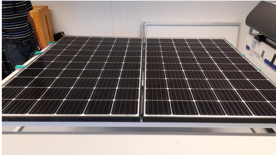
Figure 5.7: Visual inspection of the monofacial module. Left: Fielded module. Right: Reference module
