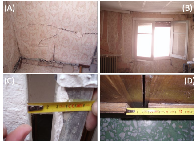
Figure 8. View of pathologies inside a Perdiguera building (6 Del Medio Street): (A) Wall cracks in the living room; (B) Cracks and deformation in a bedroom window; (C) Opening and deformation of a pile (3 cm); (D) Opening and deformation of the front door (4 cm).
