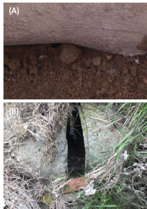
Figure 8. View of breaks in the water and sewer network of Perdiguera: (A) Crack in Del Medio Street Pipe; (B) Break in Main Collector.
