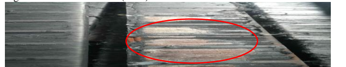
Fig. 10. Degradation of stator bar insulation.
