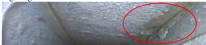
Fig. 2. Mechanical Erosion (2009) – Slot No 08 – Ventilation Channel No 01 Top Side Out.
