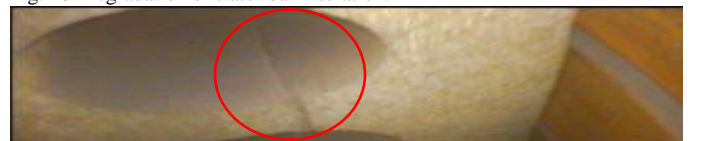
Fig. 11. Cracked Spacers Between End Windings Under Retaining Rings (2009).
