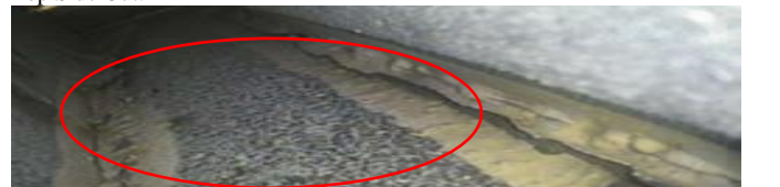
Fig. 7. Electrical Erosion (2014) – Slot No 17 – Ventilation Channel No 01 Top Side Out.
