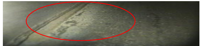
Fig. 3. Mechanical Erosion (2011) – Slot No 12 – Ventilation Channel No 05 Top Side Out.
