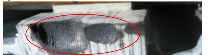
Fig. 9. Crack in Slot No 10 (2012).
