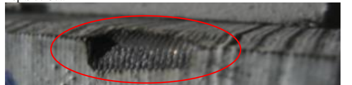
Fig. 8. Crack in Slot No 9 (2012).
