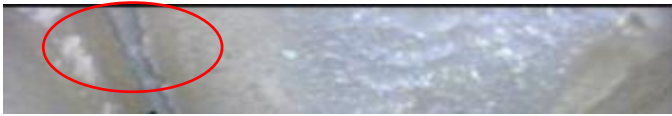
Fig. 13. Traces of slot PD (2009) – Slot No 18 – Ventilation Channel No 03 Top Side Out.
