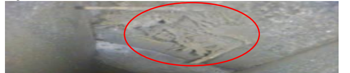
Fig. 5. Electrical Erosion (2009) – Slot No 12 – Ventilation Channel No 02 Top Side Out.
