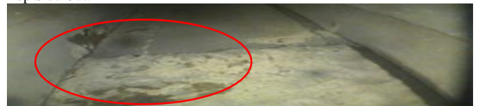
Fig. 6. Electrical Erosion (2011) – Slot No 12 – Ventilation Channel No 77 Top Side Out.
