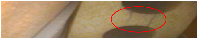
Fig. 12. Cracked Spacers Between End Windings Under Retaining Rings (2009).
