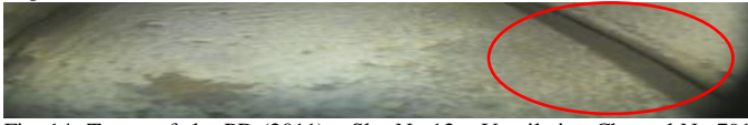
Fig. 14. Traces of slot PD (2011) – Slot No 12 – Ventilation Channel No 791 Top Side Out.
