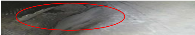
Fig. 15. Traces of slot PD (2014) – Slot No 15 – Ventilation Channel No 47 Top Side Out.
