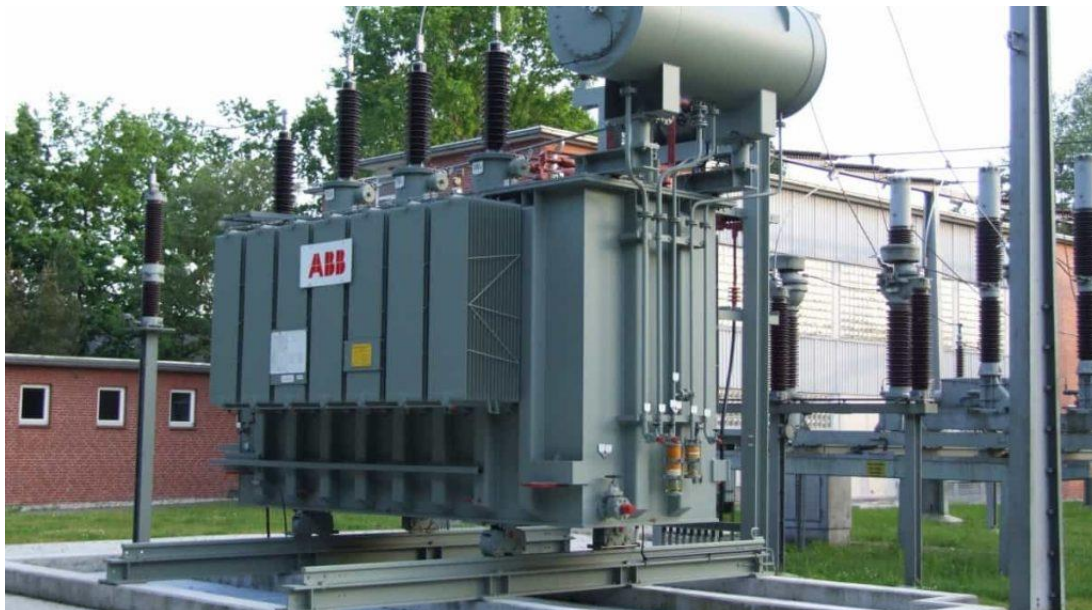
Figure 9: Example of transformer
