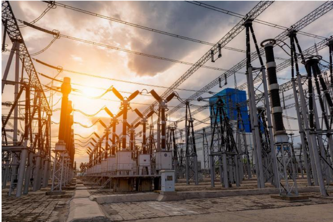
Figure 10: Image of Substation
