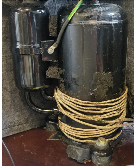
Figure 20: Placement of the heating wire around the compressor.
