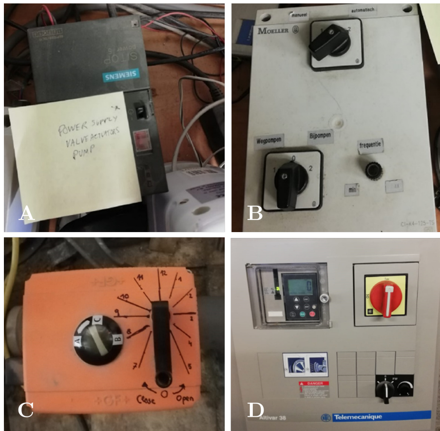
Figure 5.5: A: Power supply valve actuators pump. B: Steering pump box. C: Flow Controller. D: Local control panels of the pumps. Source: Ricci (2021).
