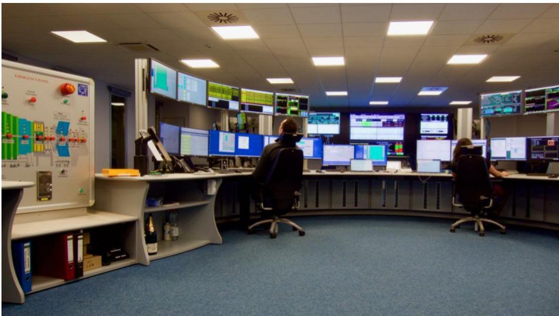
Figure 4. The LHCb control room.
