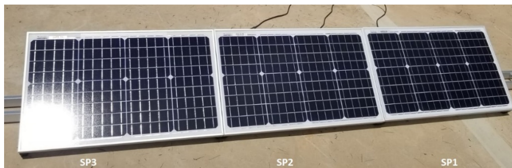
Figure 3. View of solar panels in String.
