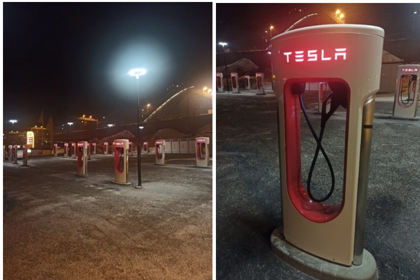
Figure 27. Pictures from Örnsköldsvik (Sweden) CI with 20 CSs, each delivering up to 250 kW.
