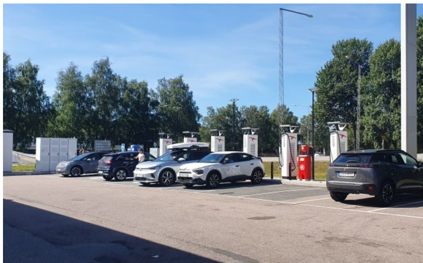
Figure 29. Ionity 350kW CSs located in Verkstadvägen – Södertälje (Sweden) [106].
