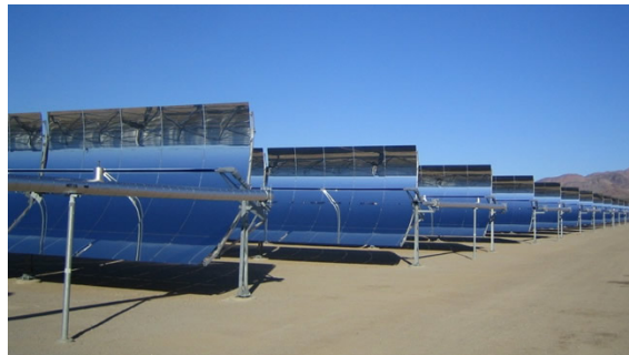
Figure 3: Parabolic trough collector. Source: Taken of Villasante2010.
