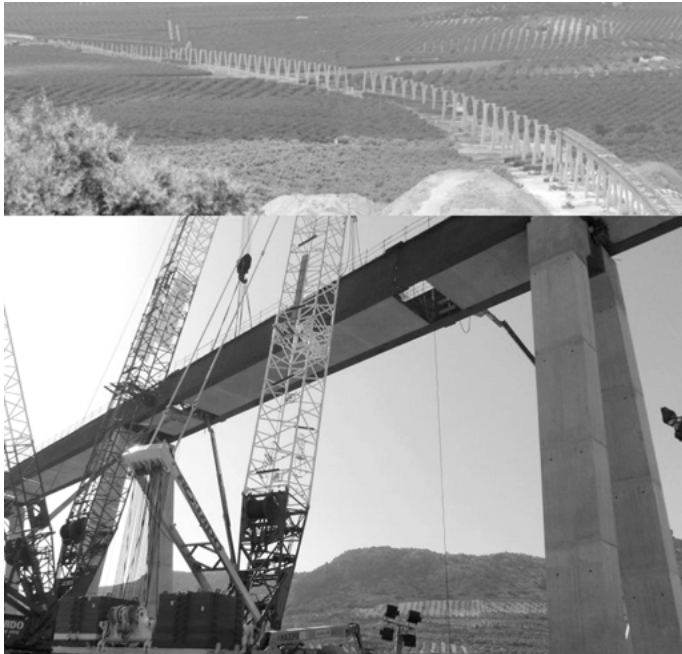
Fig. 11: Archidona (Spain) viaduct: continuous composite twin-girder bridge with upper and lower concrete decks. Image courtesy of Alejandro Castillo Linares ( http://www.acl-estructuras.com ).
