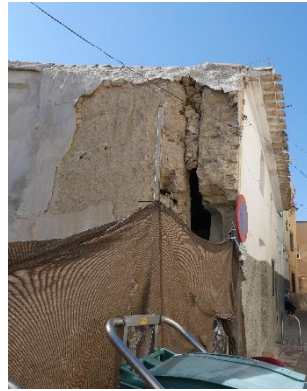
Very bad Lack of connection between orthogonal walls
