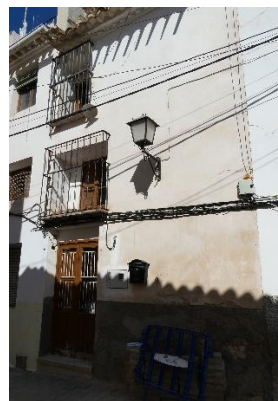
Good Small cracks in the renderings. Small stains of moisture
