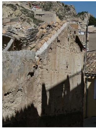
Very bad Roof and/or floors seriously damaged.
