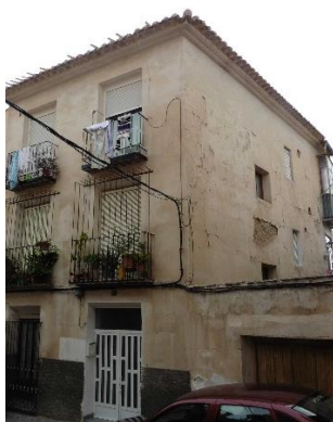
Medium Cracks in bearing walls, extended moisture in the lower part.
