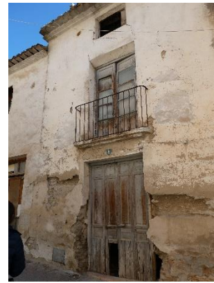
Bad Bearing walls seriously damaged
