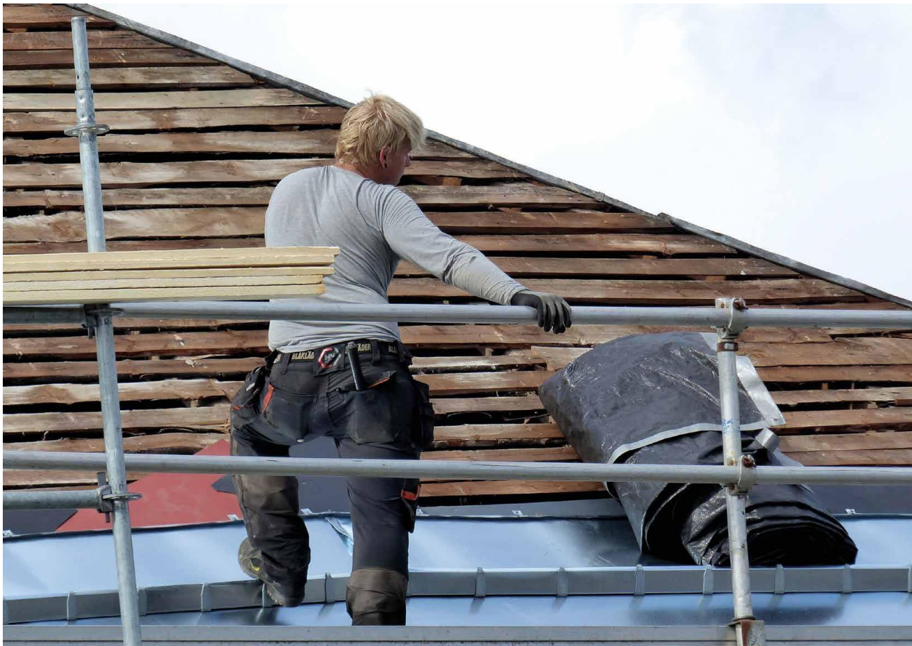
↶ Repair of a roof with a wooden board in old Rauma, Finland (© F. Vegas, C. Mileto, 2017)
