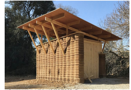
Serra Utkum Ikiz. 12/09/2022, Spain's first building made with earth and a 3D printer: TOVA
