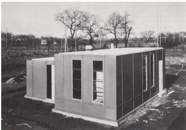
Figure 1: Stahlhaus during its construction. Source: Engelmann, Ch. and Schädlich, Ch. (1991). Die Bauhausbauten in Dessau . Berlin: Verlag für Bauwesen.
