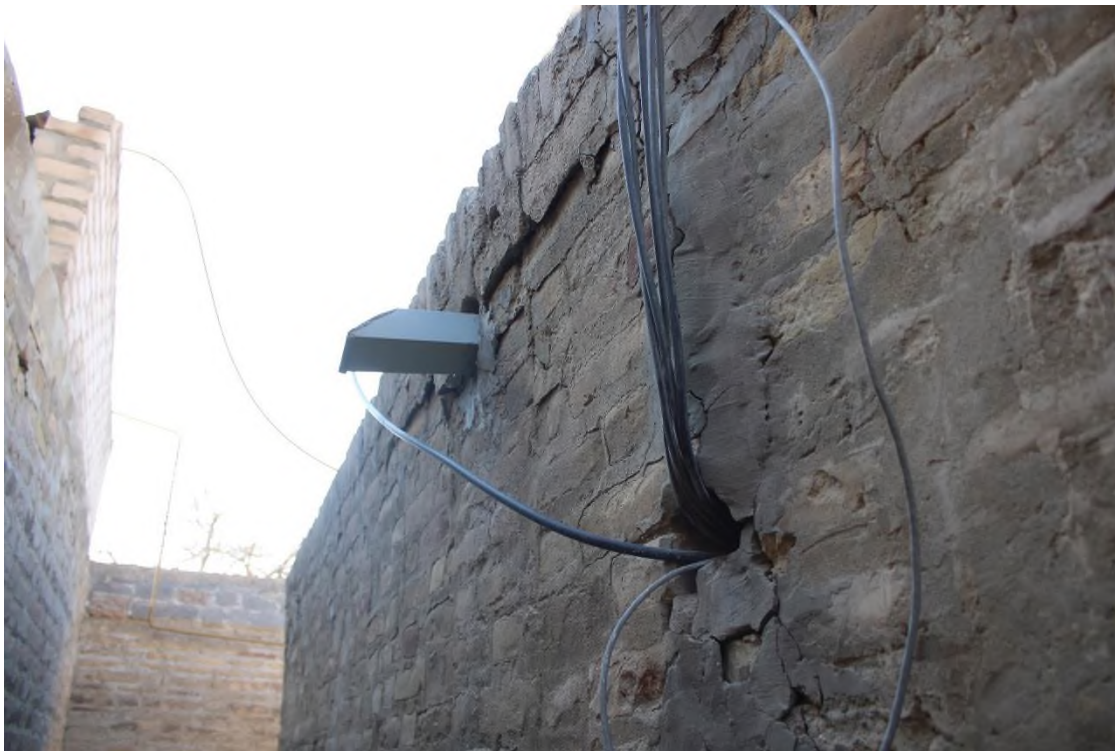
Source: Author: Walls of the Zindan. The cables are routed through the walls. Cables were laid to carry out electricity, security, cameras, and work at the cash register – Upper east side.
