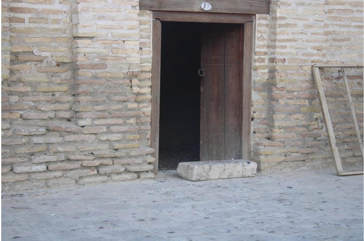
Source: Author: Walls and abandoned cells damaged by salinity and moisture
