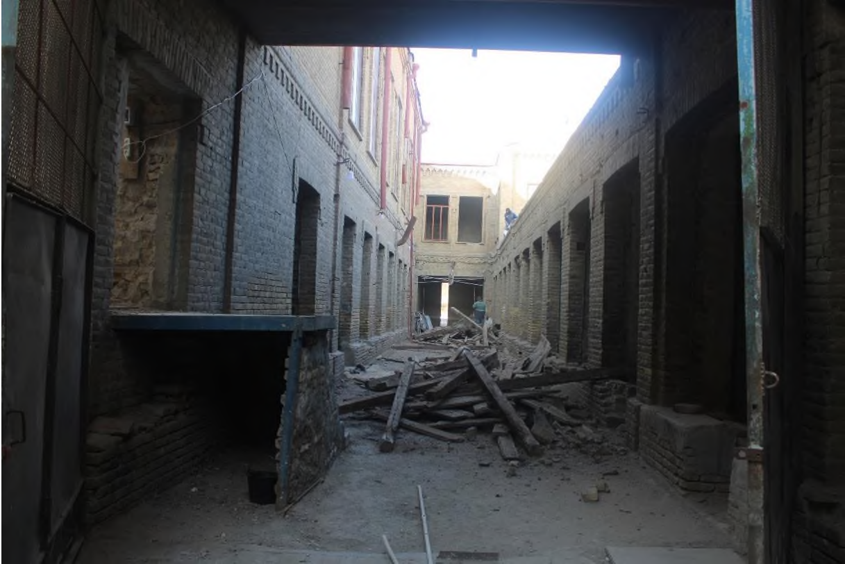
Source: Author: Inner courtyard of the Passage that reconstruction works are going.
