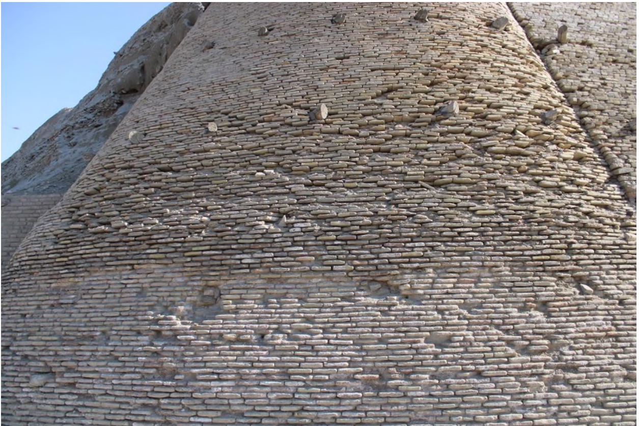
Source: Author: Heavy rains and salinity erode the wall day by day—the north-west wall of Ark.
