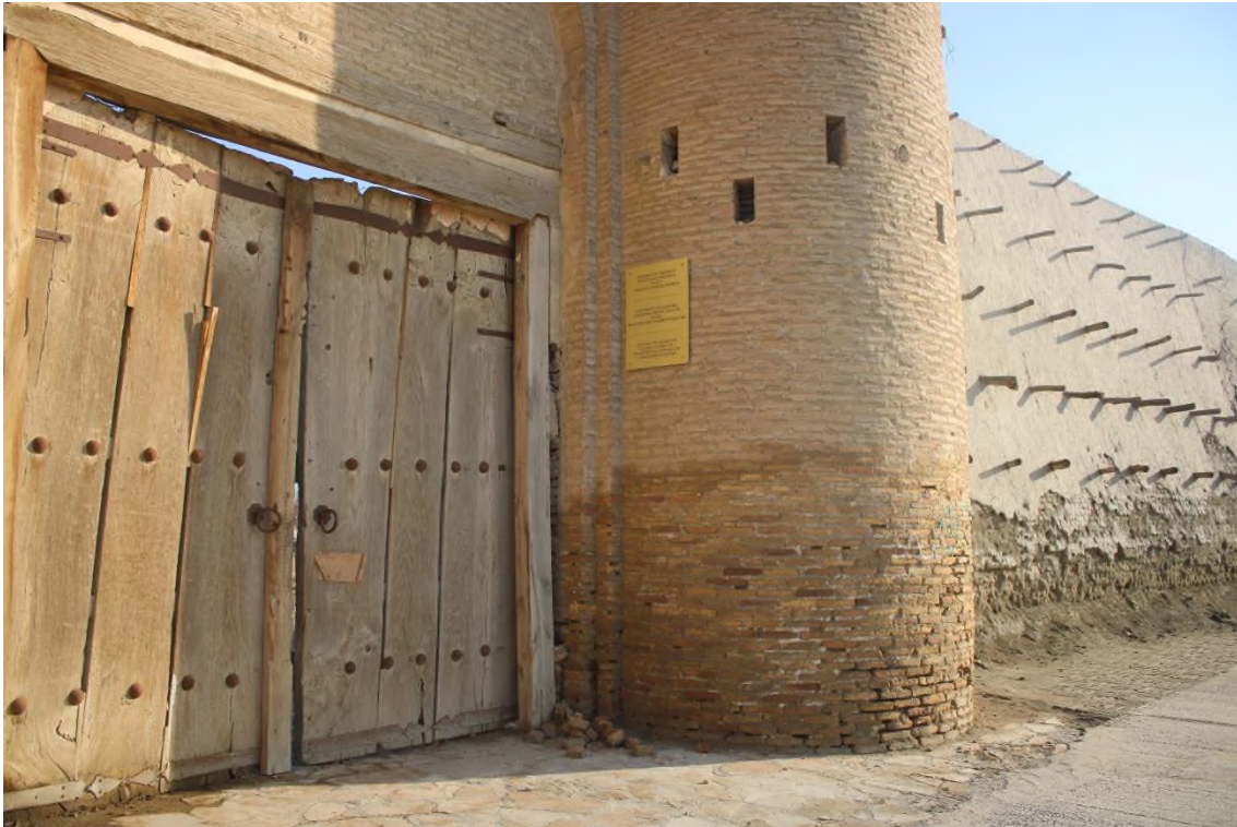
Source: Author: The Talipochgate and Wall. It is visible the salinity and humidity effect on the wall fundament
