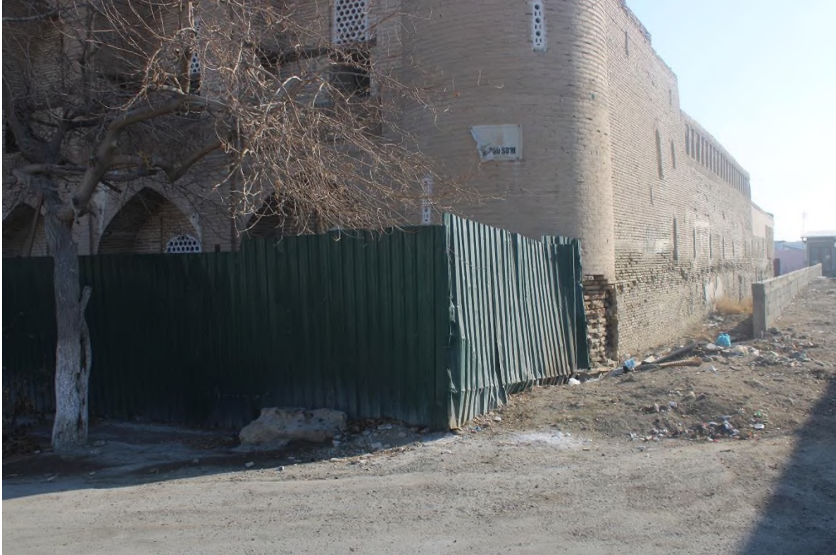
Source: Author: West part walls of the madrasah that neglected for many years. Lack of appreciation by local people.
