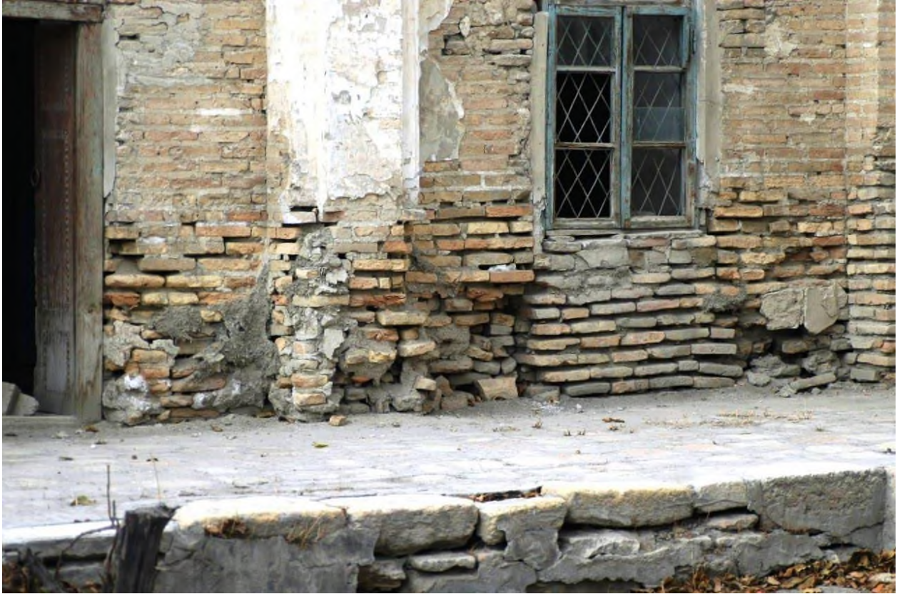
Source: Author: damaged walls
