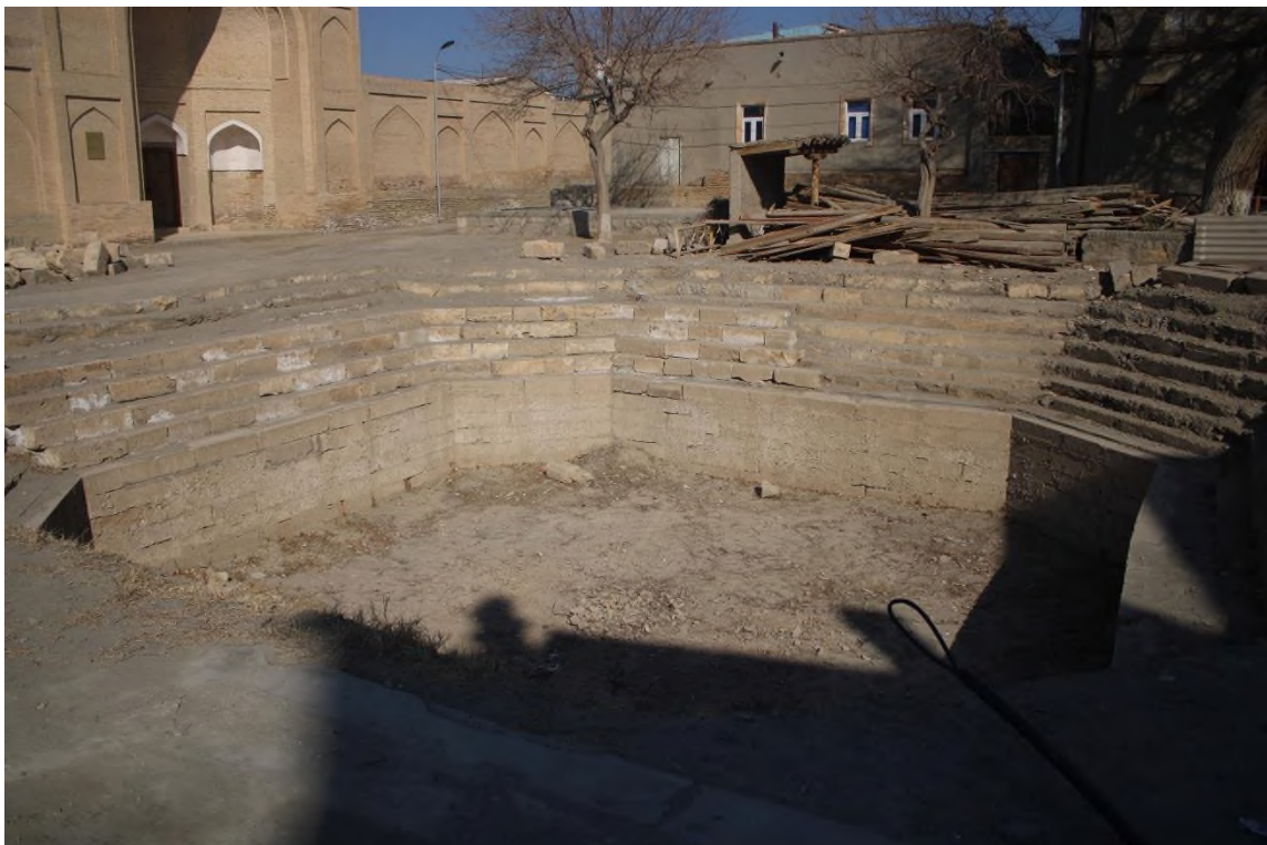
Source: Author: East side of the Minaret, restoration works is started. During the inventory it is stopped
