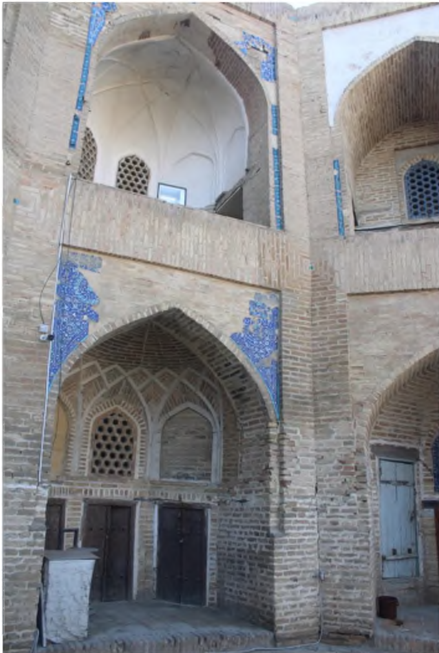
Source: Author: Damaged walls because of salinity and humidity
