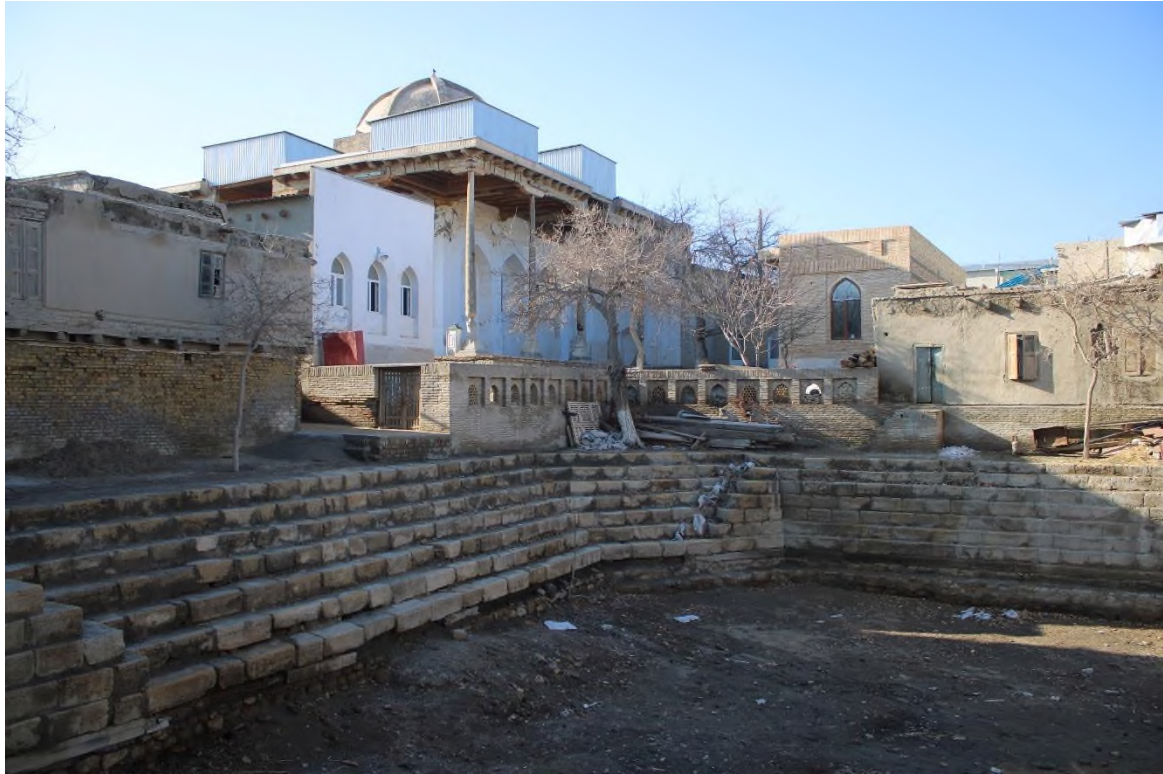
Source: Author: Hauz and Mosque (Possible to see the repairing works in Hauz section of the complex)
