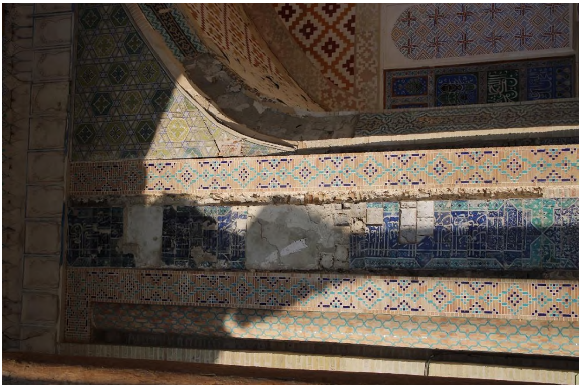
Source: Author: Damaged walls of the Mosque
