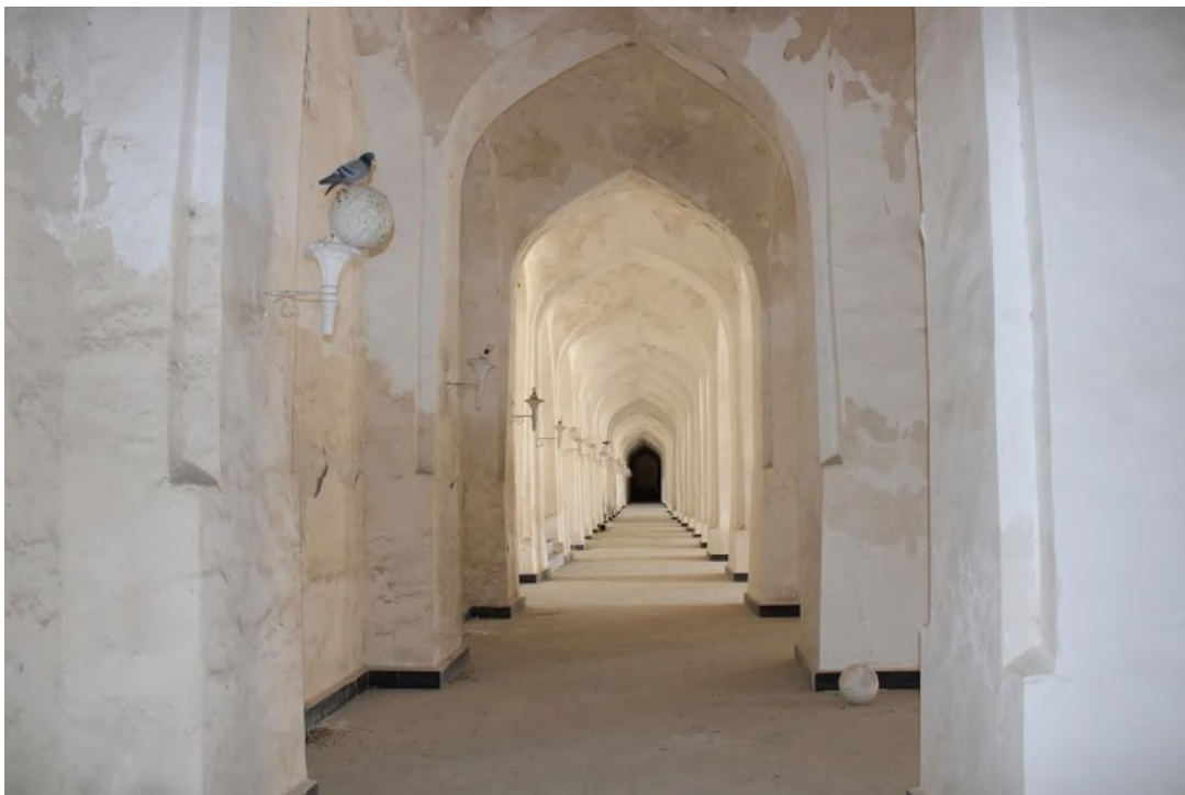
Source: Author: The decorative part of the walls separated due to the damp top
