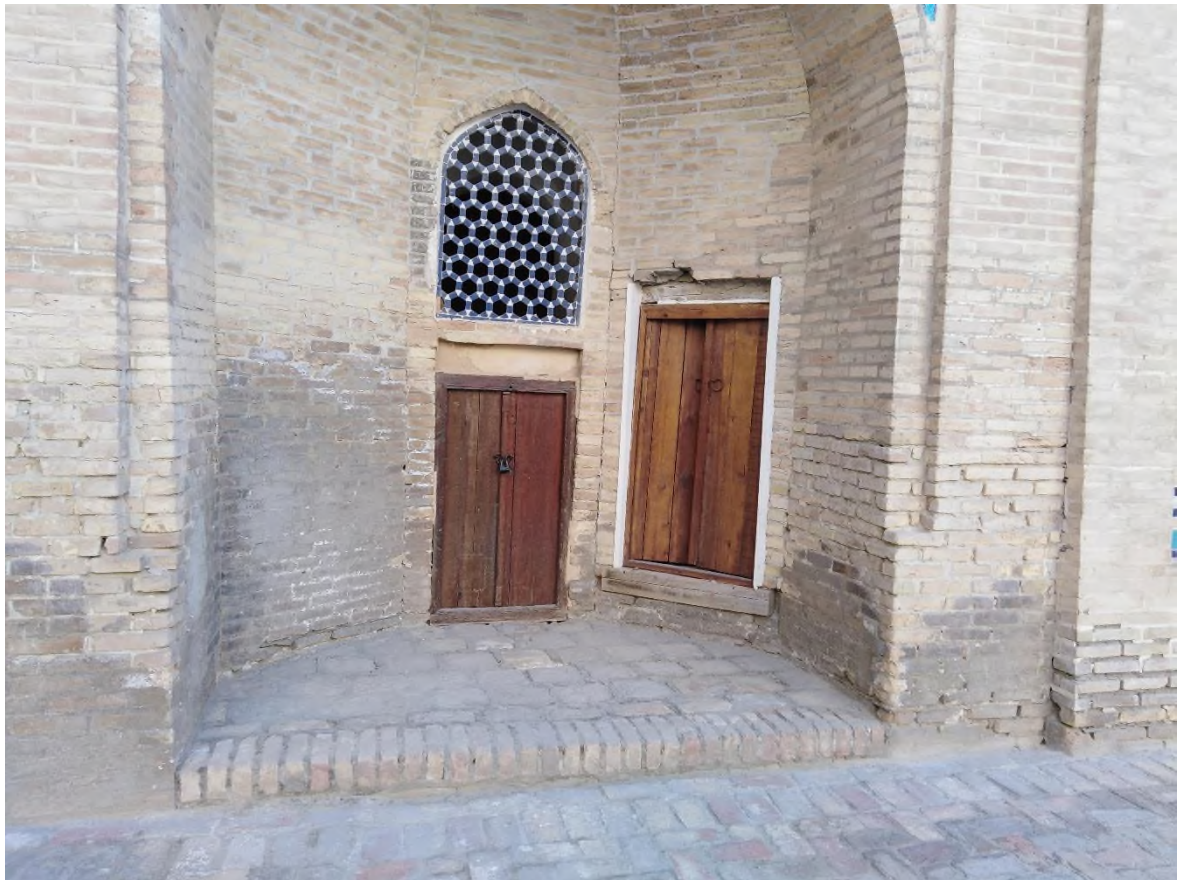
Source: Author: entrance to hujra; it is closed by NGO. Salinity and humidity affect to the building.
