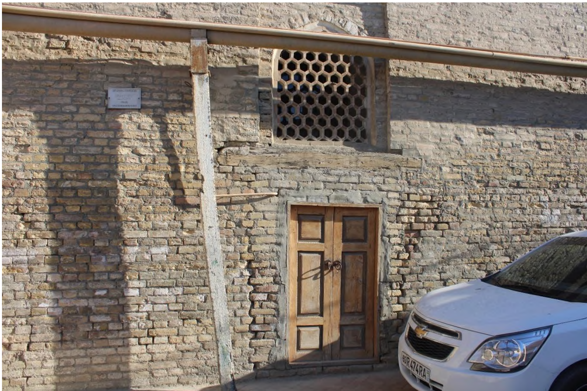
Source: Author: Old and main door of the Mosque. Now it is closed. Only entrance by inside the hotel
