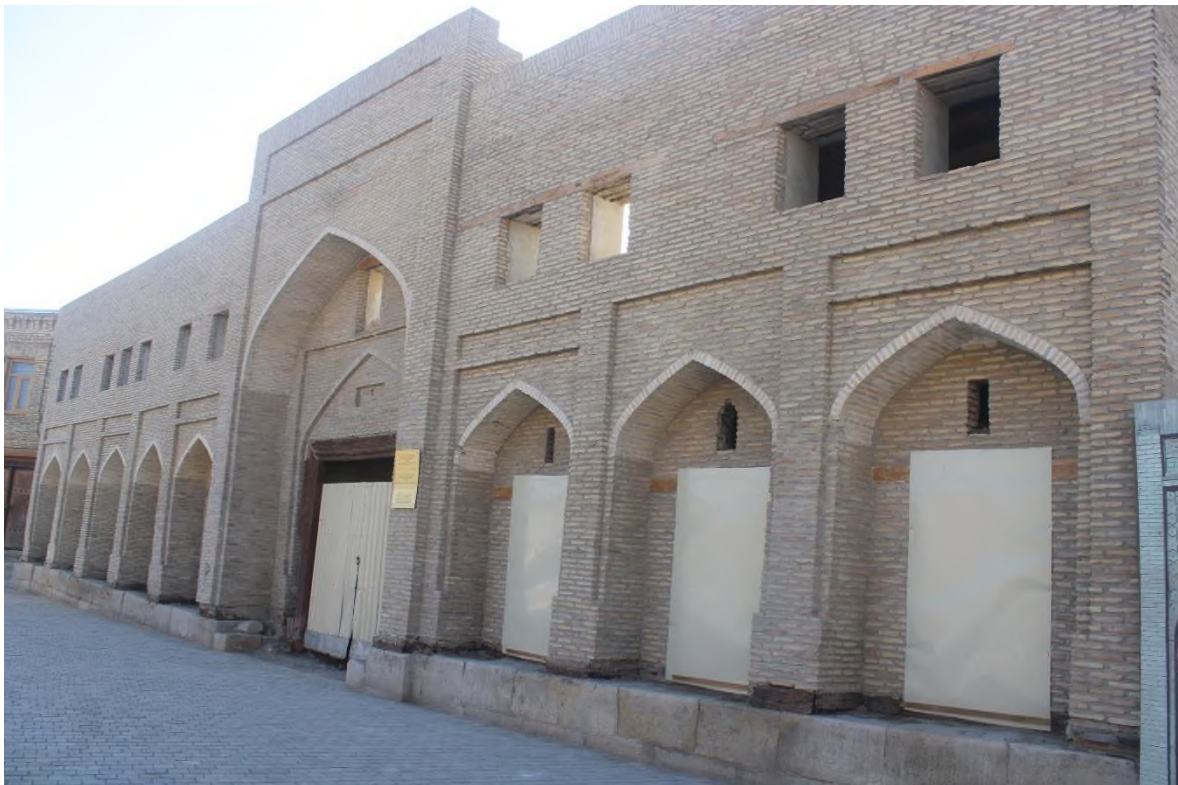
Source: Author: Rashid caravansarei. It is closed. Construction works in going inner part of the heritage
