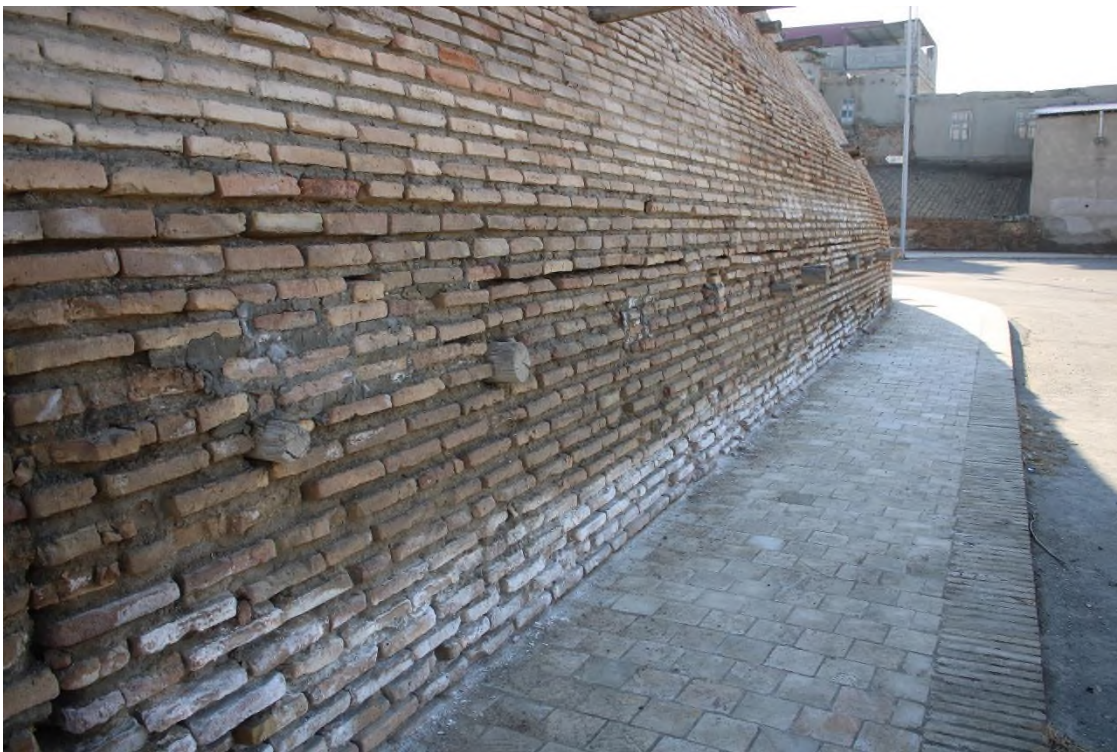
Source: Author: The foundation walls of the Zindan - Moisture and salinity hit the walls
