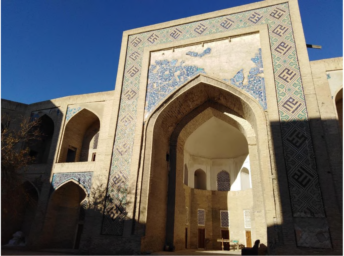
Source: Author: west part of the Madrasah needs preservation works.
