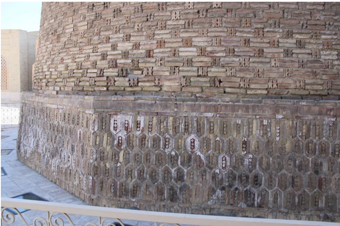
Source: Author: Possible to see the effect of salinity on the fundament of Tower.
