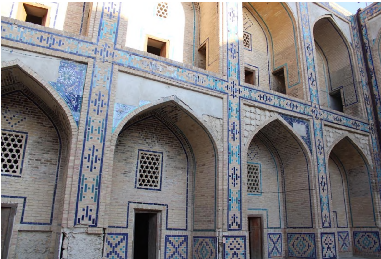
Source: Author: walls of the masrassah, it need preservation works.
