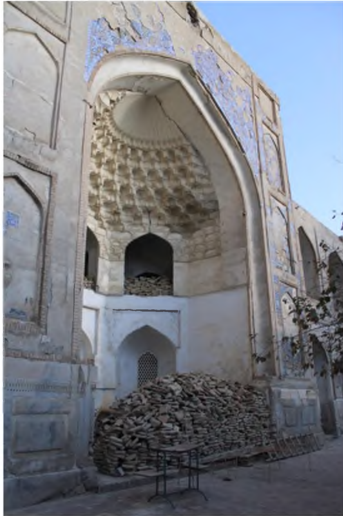
Source: Author: Eastern part. It needs capital restoration.
