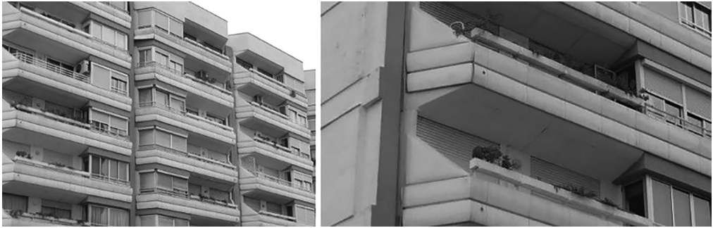
Figure 11. General view and detail of the front of the Paz y Seguridad Building. The earlier composition of the Ciudadela Building is repeated in the image of this group. The bulging polyester profile of the modular boxes provides lightness and distinguishes it from the earlier building. It can be seen that the plant boxes are free-standing outside the Modular Boxes. Modulares. Valencia. GO.DB. Architects. (Photo: Maite Palomares, 2009. Private Archives of Maite Palomares.)
