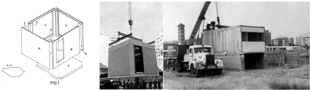
Figure 3. M-IV Modular Element. Mounting the panels and special elements required for the joints. Raising an M-IV for positioning on site and the composition of three M-IV to form a habitable beam, of rectangular proportion. In this case, the building of housing in Camapanar is shown with the lower number of joints compared to the EM-III. (Photo collage copyright of the authors.)
