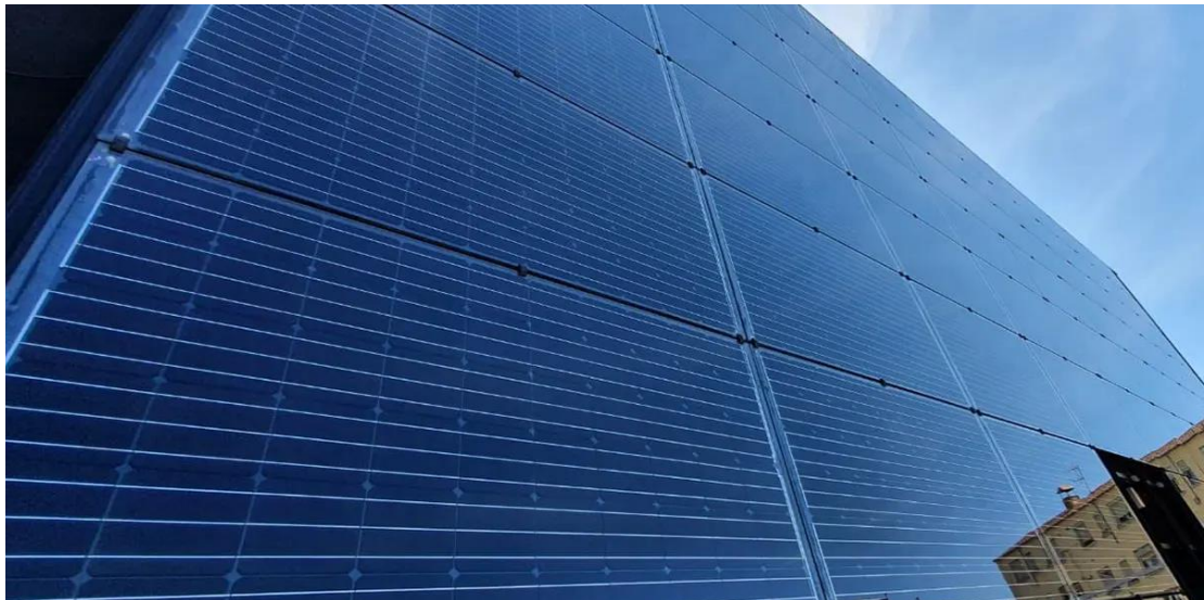
Figure 8. Façade of a BIPV installation. [15]
