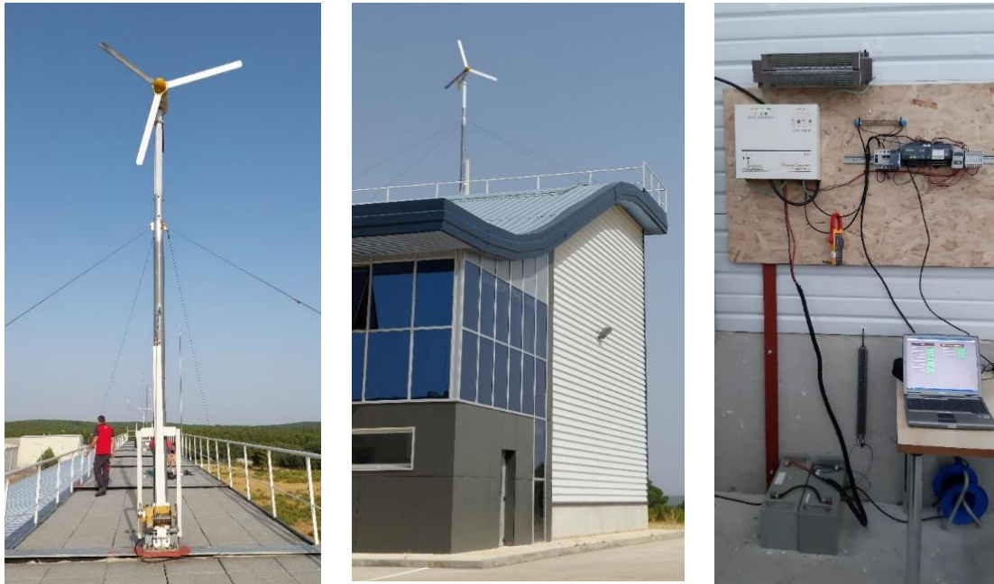
Figure 10. Small wind turbine installation at roof lab and measuring board
