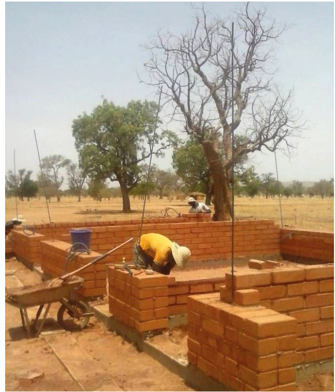
Construction of walls with compressed earth blocks reinforced with rebars in joints and jambs.
