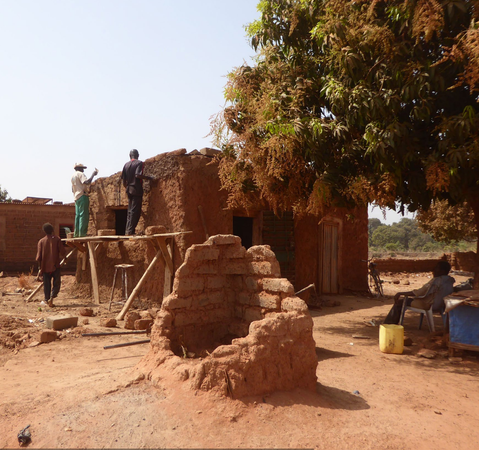
Maintenance proceeds for a dwelling, with the repeated rendering of walls with mud.
