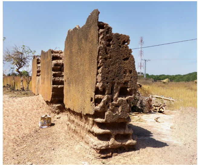
A case similar to the previous one, causing more damage to the lower sections of the wall.
