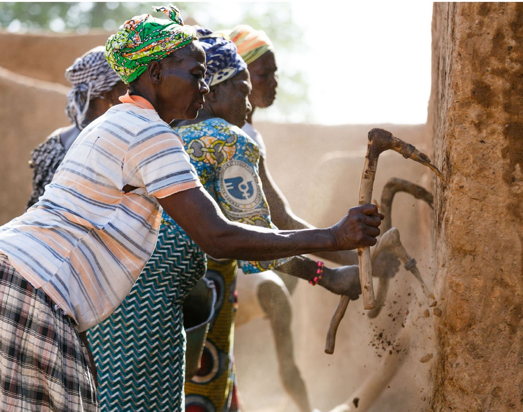
Kassena women chiselling off the old rendering before applying the new one.
