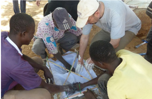
Construction of the frame, putting the fabric in place and soaking it in gypsum.
