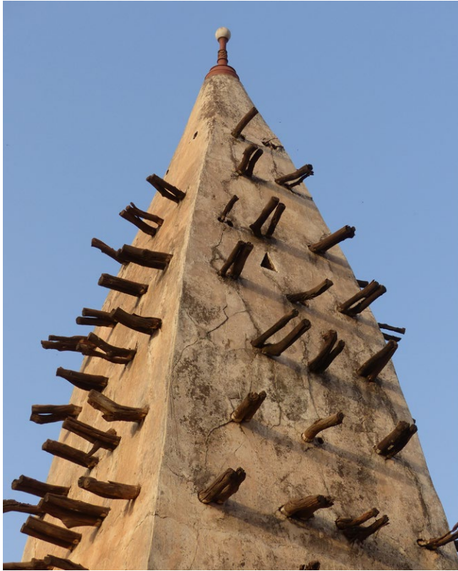
Tower of the Bobo-Dioulasso mosque bristling with sticks and branches used to periodically climb and repair the mud rendering.
