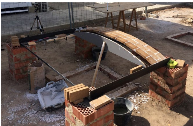
Complete CEB tile vault and tests for the construction of small wall partitions to support the paving.
