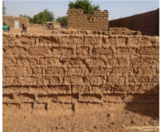
The damp in the ground, worsened perhaps by the presence of cement in the joint mortar, is causing erosion in the adobe bricks most in contact with the ground.
