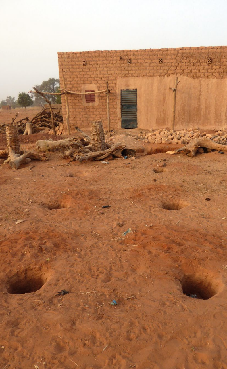
Holes made in the ground for the foundation of the wooden posts.
