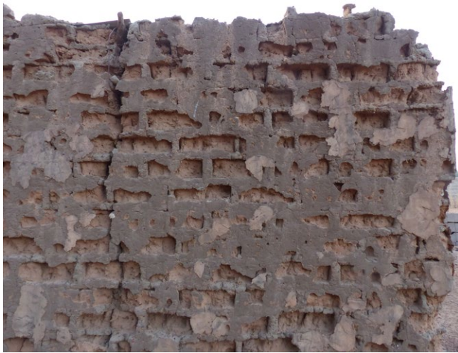
Joints and cement mortar rendering on the adobe wall which is gradually wearing down the body of the earthen wall, due to incompatibility between the two.
