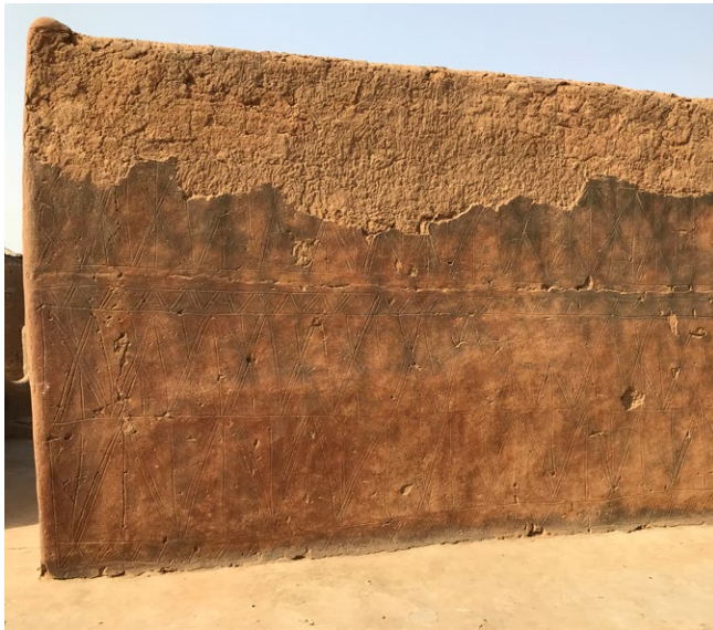
Detachment of the carved and painted rendering of a house of the Royal Court of Tiébélé, probably due to the damp caused by rain.
