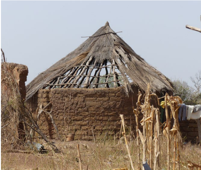
Poor maintenance of a thatched roof, leaving the adobe construction exposed to rain and therefore at risk of collapse.
