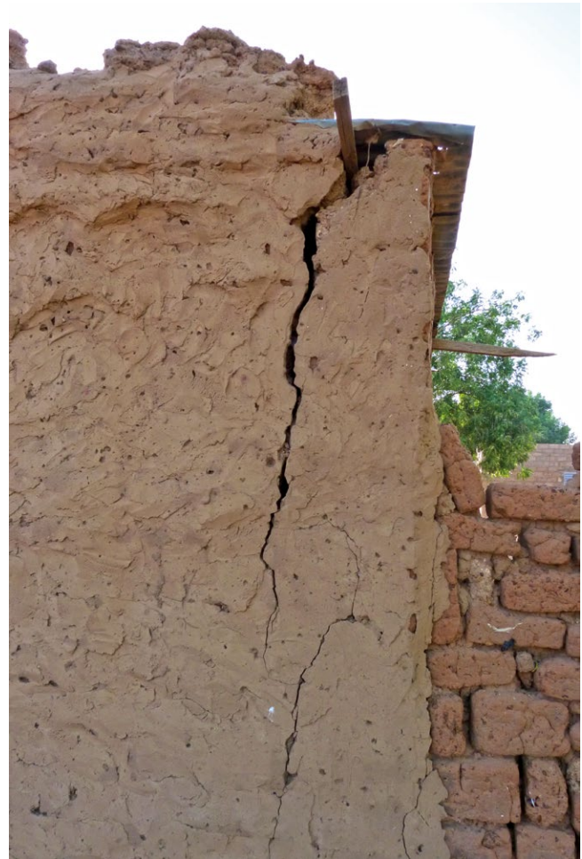
Crack on a corner caused by a poor connection between the two converging walls.
