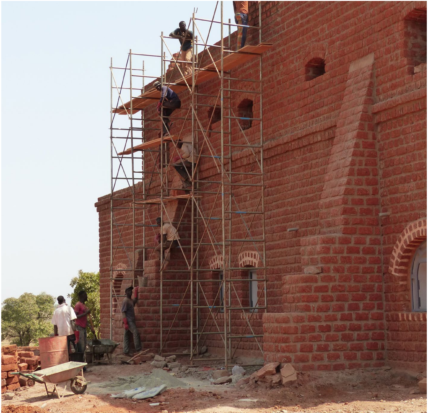
Construction of the Shea Research Centre in Satiri, Bobo-Dioulasso (Burkina Faso), designed by Chiara Rigotti.
