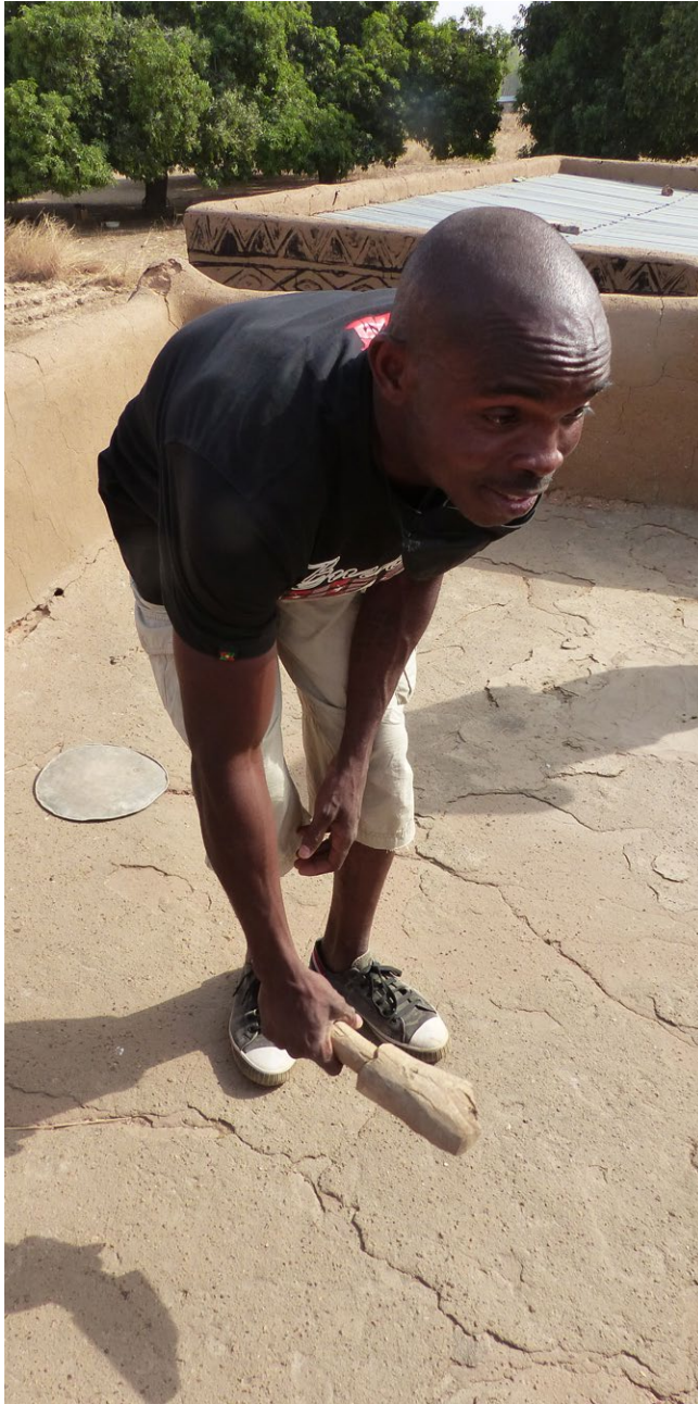
Example of the system for tamping the earth of the flat roofs of Kassena dwellings repairing them with a rammer.
