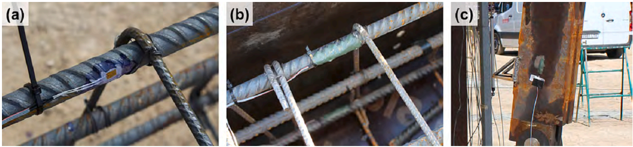
Fig. 5. (a) Strain gauge placed on column reinforcement before applying protective covering putty; (b) Strain gauge placed on column reinforcement prior to concreting; (c) strain gauge placed on collapsible steel column.
