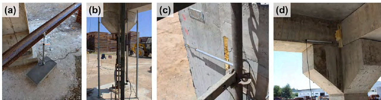
Fig. 8. Displacement transducer used to monitor: (a) vertical settlement of foundation, (b) vertical displacement of first floor, (c) building drift (connected to detached auxiliary structure), and (d) horizontal contraction at the bottom of beam-column joint.
