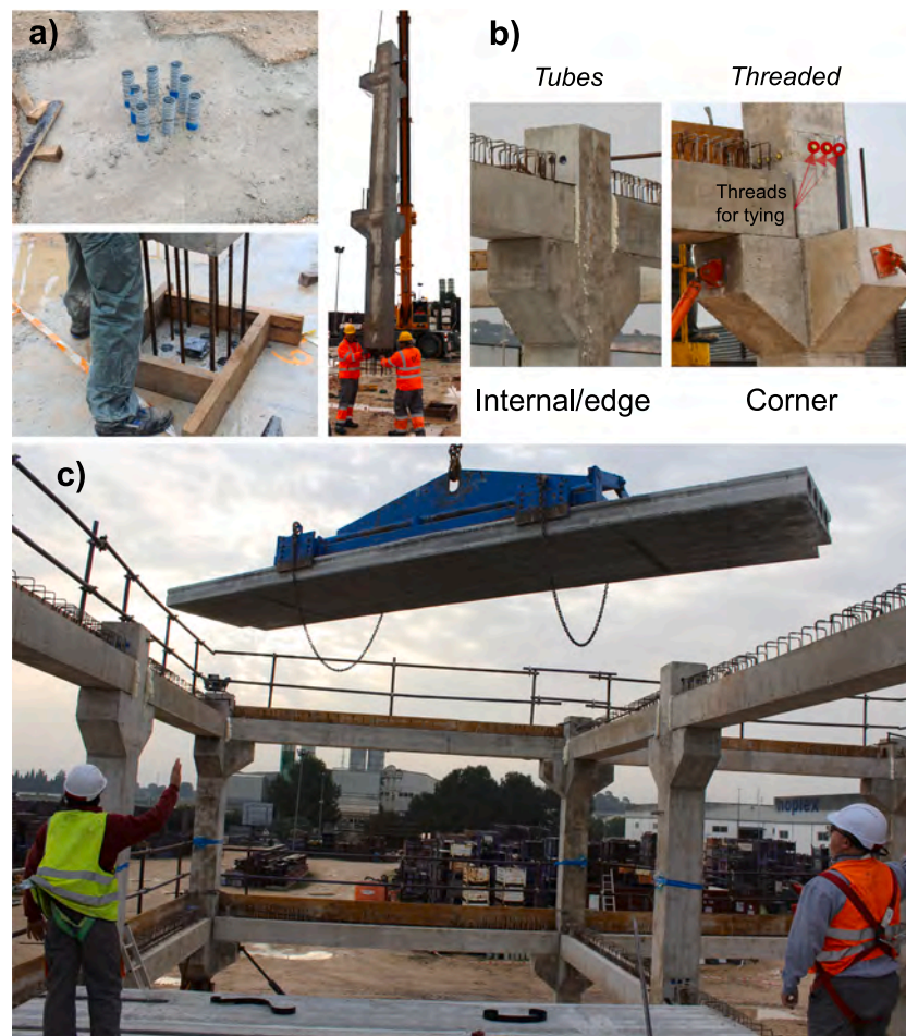
Fig. 2. Details of the building during construction: foundation (a), connections prepared for ties in edge, internal and corner columns (b) and placing of hollow-core units for the slabs (c).
