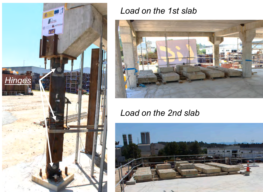
Fig. 4. Steel column designed for the sudden removal and load superimposed on the 1st and 2nd slabs.
