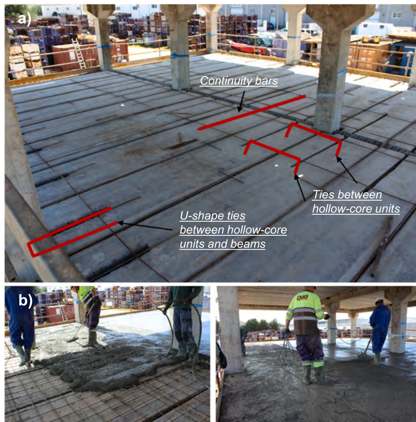
Fig. 3. Details of the slab ties and continuity bars (a) and concrete topping on the slabs (b).
