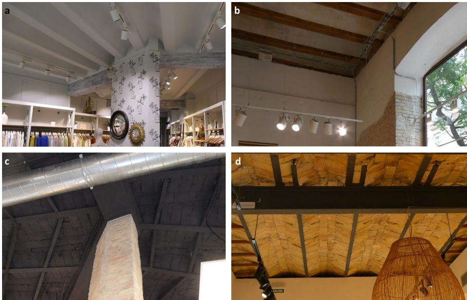
Fig. 14 Structural typologies: a timber beams and joists, b brick masonry bearing wall and timber joists, c brick masonry column with steel beams and joist and d steel beams and light tiles vaults. (Source: Authors 2021–2022)
