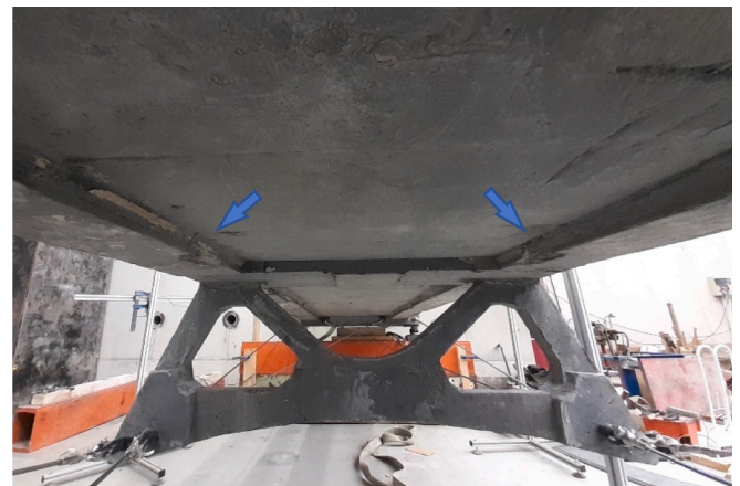
Fig. 22. Localized defects in the bottom face of the deck.
