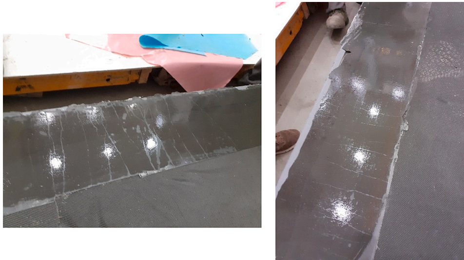
Fig. 23. Smeared cracks along the upper face of the deck. Left: concentrated cracks at the localized weaker cross-section; right: smeared cracking pattern along the upper face of the deck.
