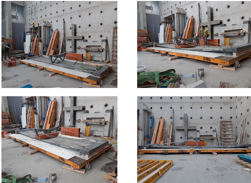
Fig. 18. Activation process. Upper-left: the structure after unmoulding (the external cables bear no tension); upper-right: the structure resting on lateral supports made of wooden blocks, loaded in the centre (note the slack cables); lower-left: external cables have been shortened in preparation for the first unloading step; lower-right: pre-deformed structure with cables in tension after full removal of the activation load.
