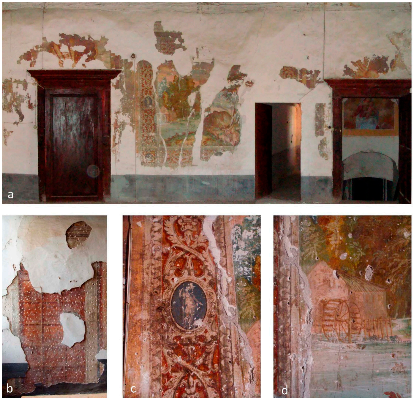
Figure 20. Details of the mural paintings and doors of the central hall on the first floor: (a) general view of the west wall of the hall; (b) detail of the fake door; (c) detail of the molding of one of the boxes; (d) detail of a watermill painted in a landscape.
