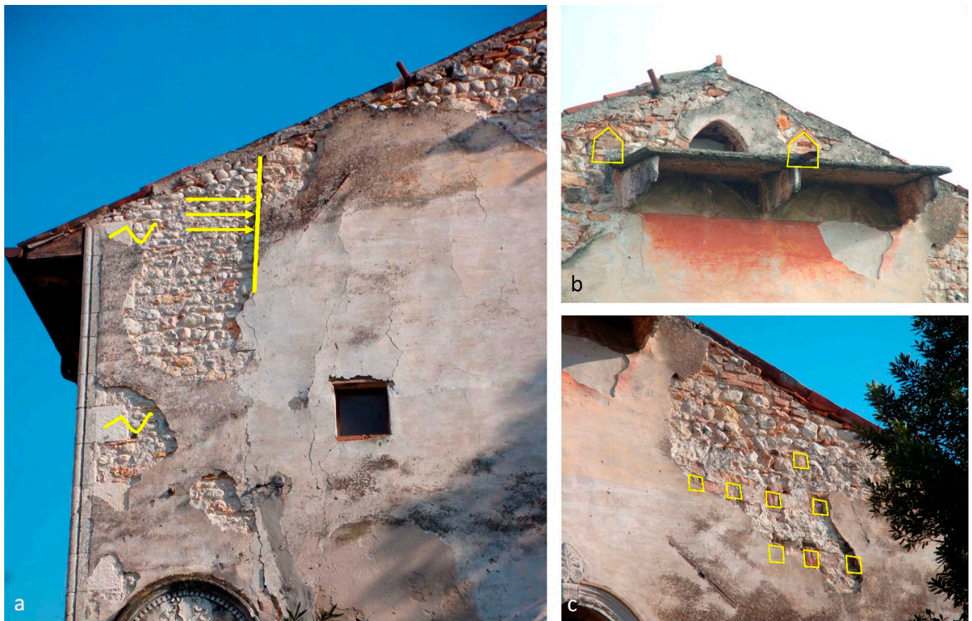
Figure 8. Detail of the west façade of the palace: (a) the structure of the staircase rests on the former corner of the building: The contemporaneity between the corner and the fabric is visible (highlighted with the symbol ~) and how the same fabric is attached to a pre-existing corner (marked with the symbol ←); (b) lunettes of the trompe l'oeil mullioned window and small blocked-off windows; and (c) blocked-off windows of the dovecote tower.
