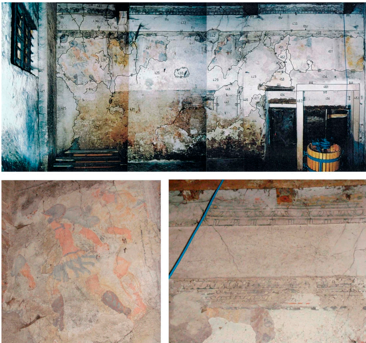
Figure 15. General view of the east side of room B6 and detail of frescoes.
