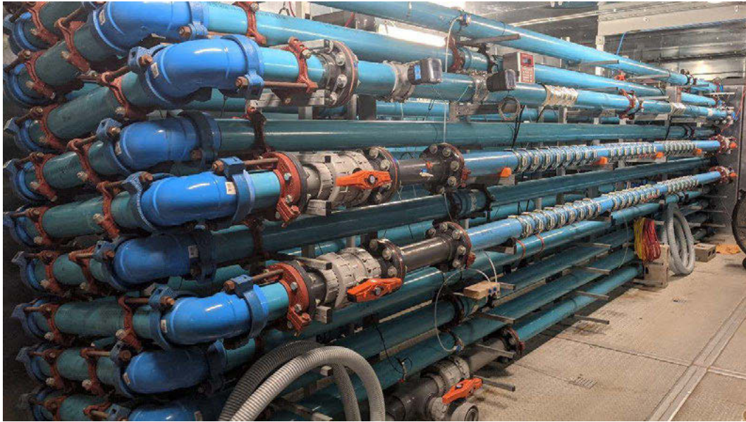
Figure 1. Drinking Water Distribution Laboratory (DWDL) at Queen's University.
