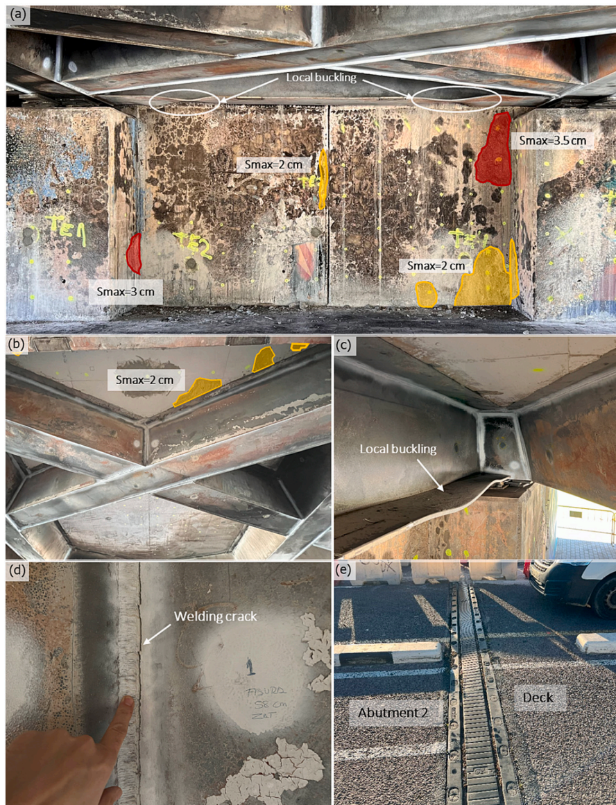
Fig. 4. Post-fire visual inspection of the bridge. (a) Overall view of the most damaged area indicating maximum spalling ( S_{max} ) in Abutment 2 as well as the diaphragm girder main damage. (b) Concrete deck spalling and overall view of out-of-plane displacements. (c) Detail of local buckling on diaphragm girder. (d) Detail of welding crack, (e) Detail of deck uplift movement noticed by the inclination of the expansion joint.
