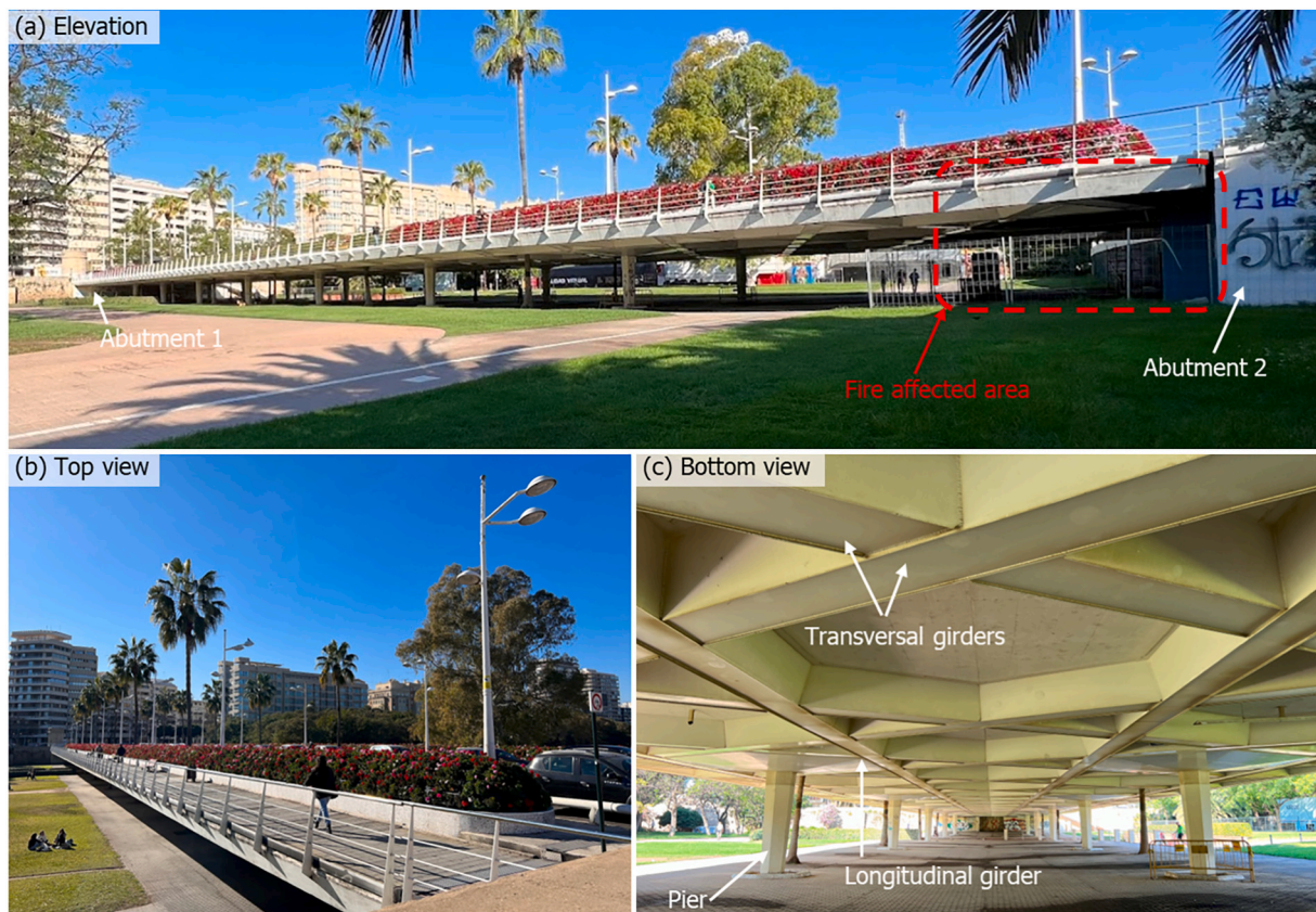
Fig. 1. Views of the “Puente de las Flores” showing also the area affected by the fire. Elevation (a), top (b) and bottom (c) views of the “Puente de las Flores”.
