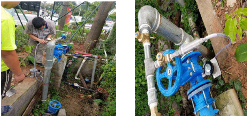
Figure 5. Pressure gauge installation at critical node
