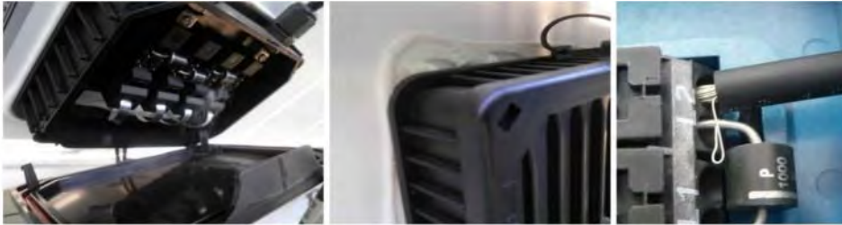
Figure 47. Junction Box Failures. a) Open JB b) Poor fixing JB c) JB with Poor Wiring (75).
