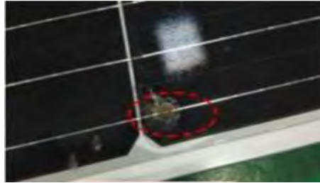
Figure 35. Hot spot in a PV Panel Surface (67).
