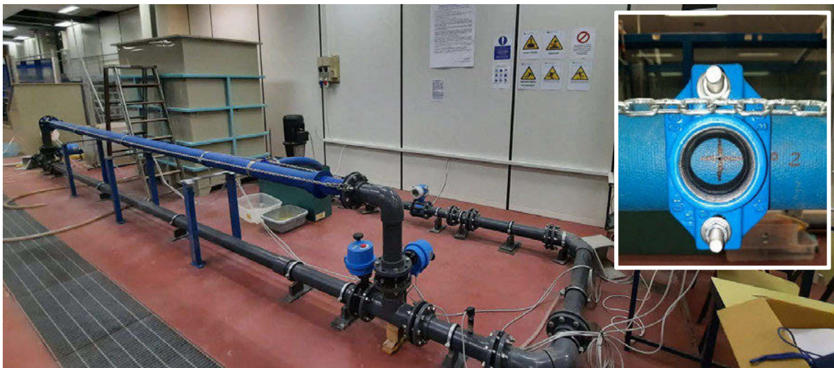
Figure 3. View of the hydraulic system after modifications; particular of the cast-iron pipe with hole used in the experiments (box on the right)
