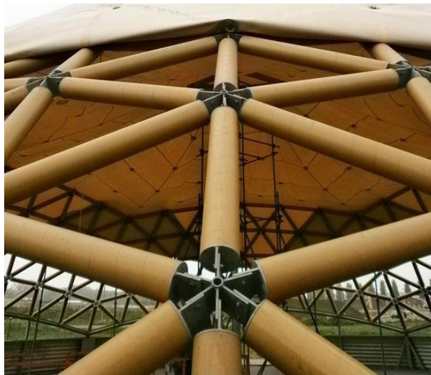
Figure 94 Picture showing Shigeru Ban's paper tower made of carton tube space frame 108
