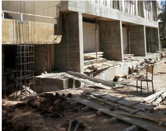
Figure 26 Picture showing a typical active construction site used by the Syrian refugees 32
