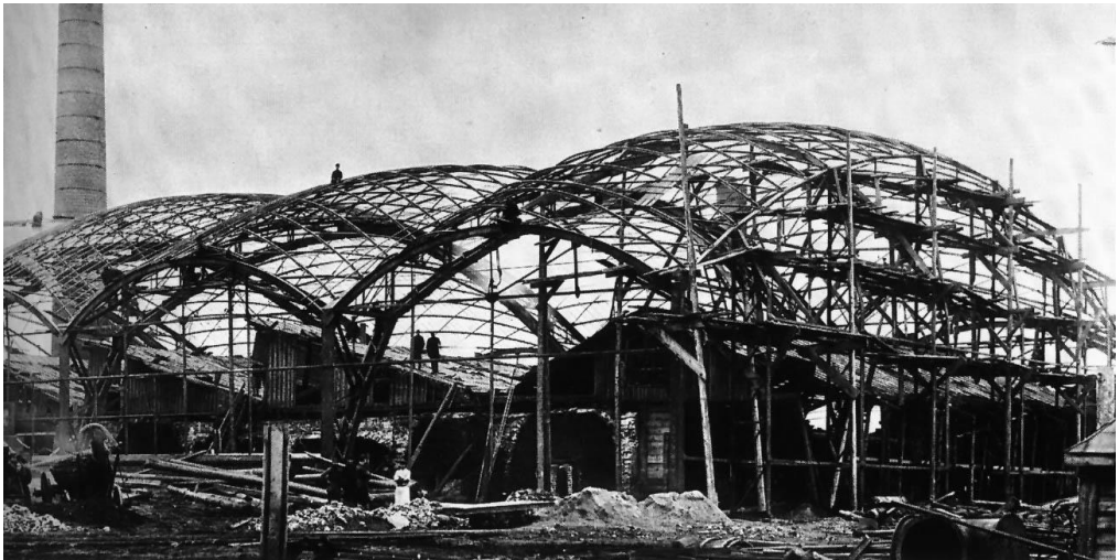
Figure 49 The double curvature Diagrid Shell by Vladimir Shukhov in Vyksa near Nizhny Novgorod during construction, 189763
