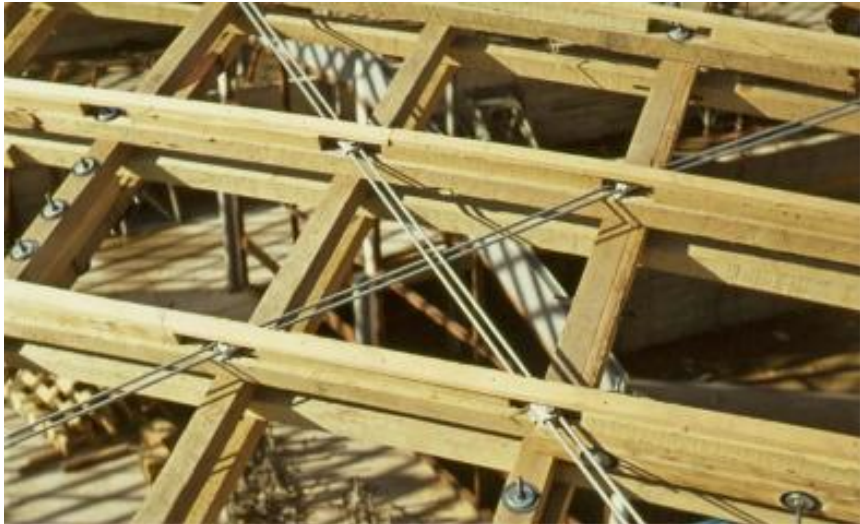
Figure 67 Picture showing the cables at the nodes 81
